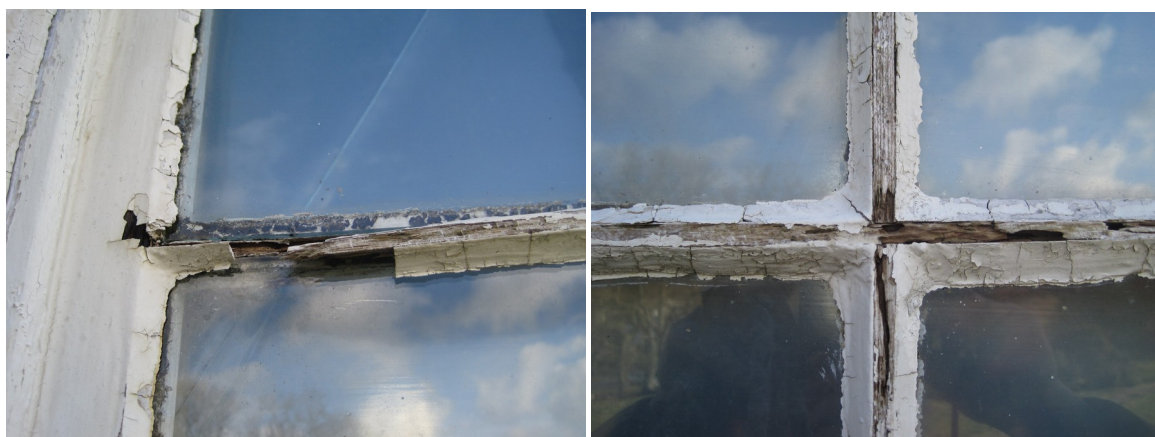
Detail of the glazing bars – which must bear the brunt of winds up to 100mph
